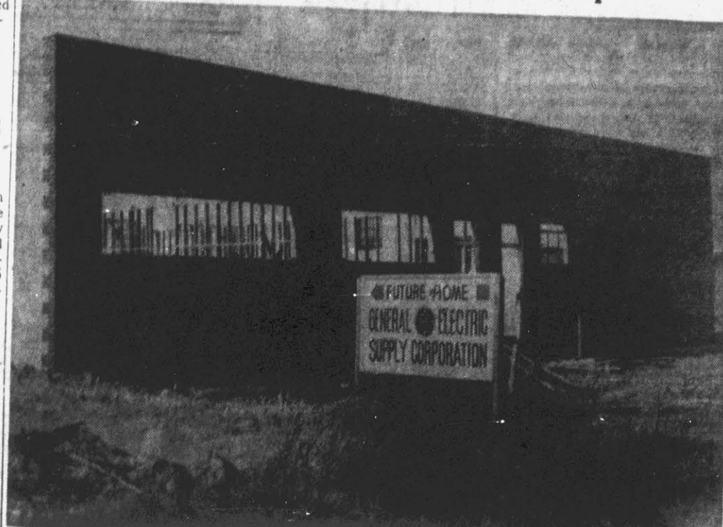
The new General Electric Supply building under construction will serve General Electric dealers in this section of the state. Construction began about 60 days ago and the building is expected to be ready for occupancy by January 25. It is located on Hooker Road. (Staff Photo by Roy Hardee).
