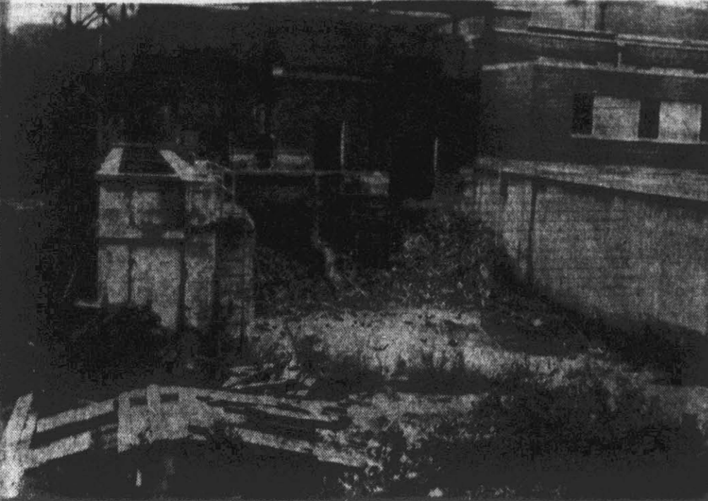
A new three-story building will be constructed in the center of this picture of the water plant here. Funds for labor on the job were approved by the Utilities Commission in a called meeting last night. Shown on the left is the original mixing chamber and on the right is shown a portion of the new settling basin that was placed in operation in 1948. Eventually the mixing chamber will be enlarged to handle three-million gallons daily. (Staff photo by John Spinks, Jr.)
