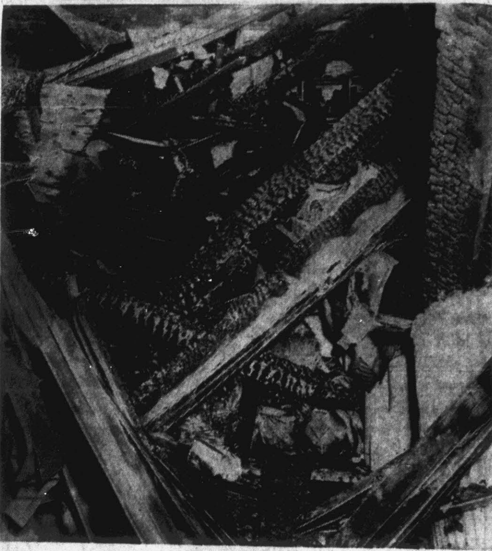
The main floor of the J. A. Watson Hardware Company is shown covered with wreckage from a fire which destroyed the roof of the building early Saturday night. While the entire roof will have to be replaced on the building, it was not believed that much damage was caused to the main floor by fire, other than water damage. The fire was believed to have originated on a platform in the back section of the building. (Reflector Staff Photo by Roy Hardee).
