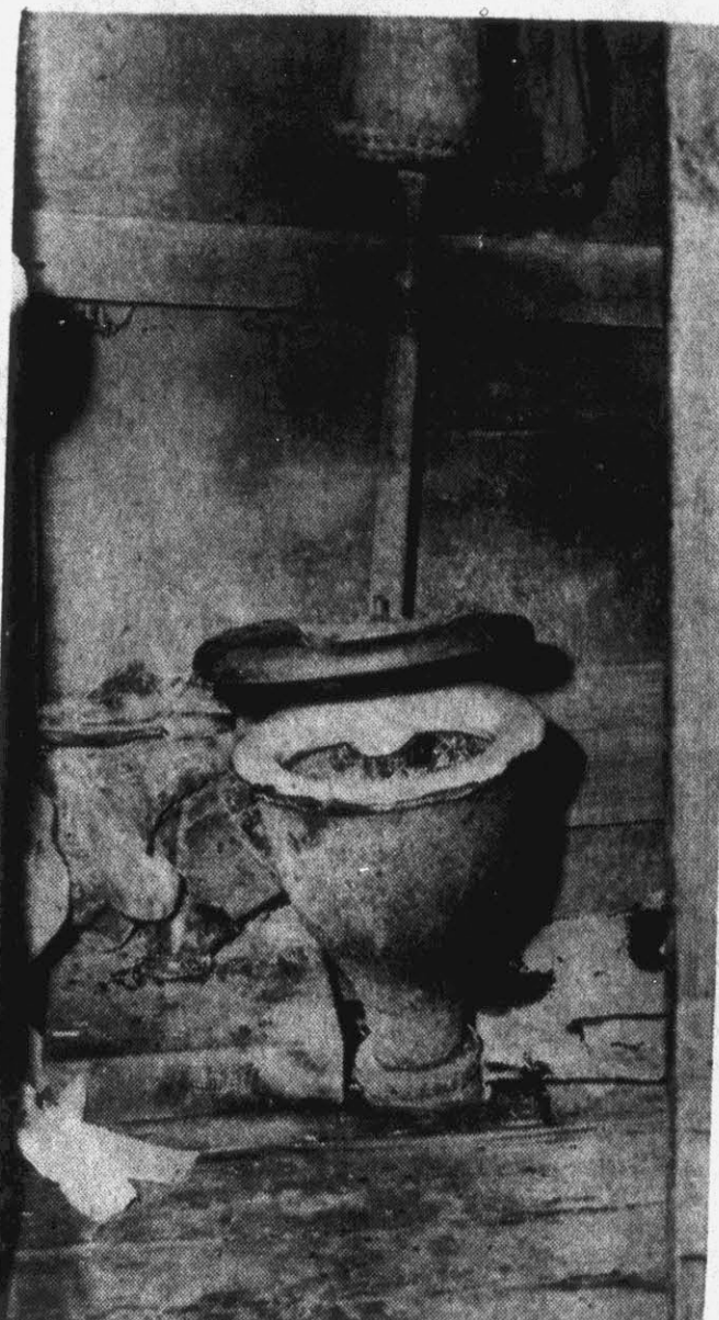
Here is one of Greenville's "modern, sanitary" privies which supposedly was to have been inspected and passed in the 1948 inspection drive held in the city. Yet this unit is in a terrible condition and does not properly operate at times. A family of four uses this unit, which is attached to the house, about five feet from the back door of the kitchen.
