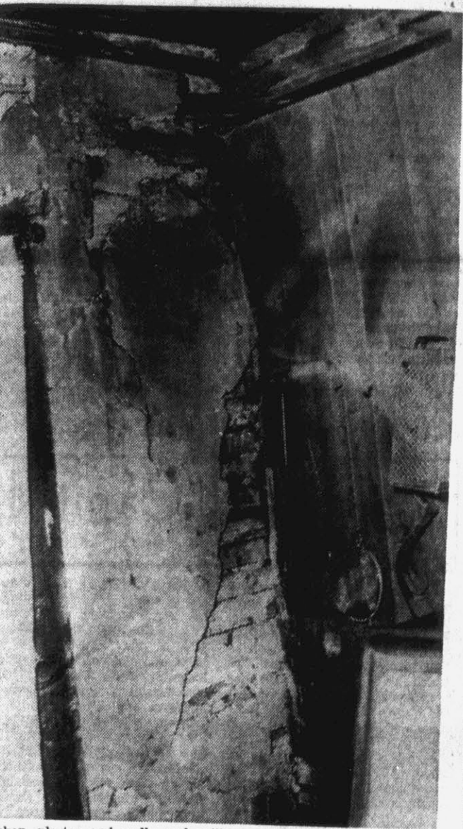
Broken plaster and walls and ceilings which are ready to come crashing down, such as the one above, are to be found all over Greenville. Tenants say that landlords refuse to do anything about these conditions, telling tenants to move if they don't like them. The picture above was made in the kitchen of a house in the river section of town.
