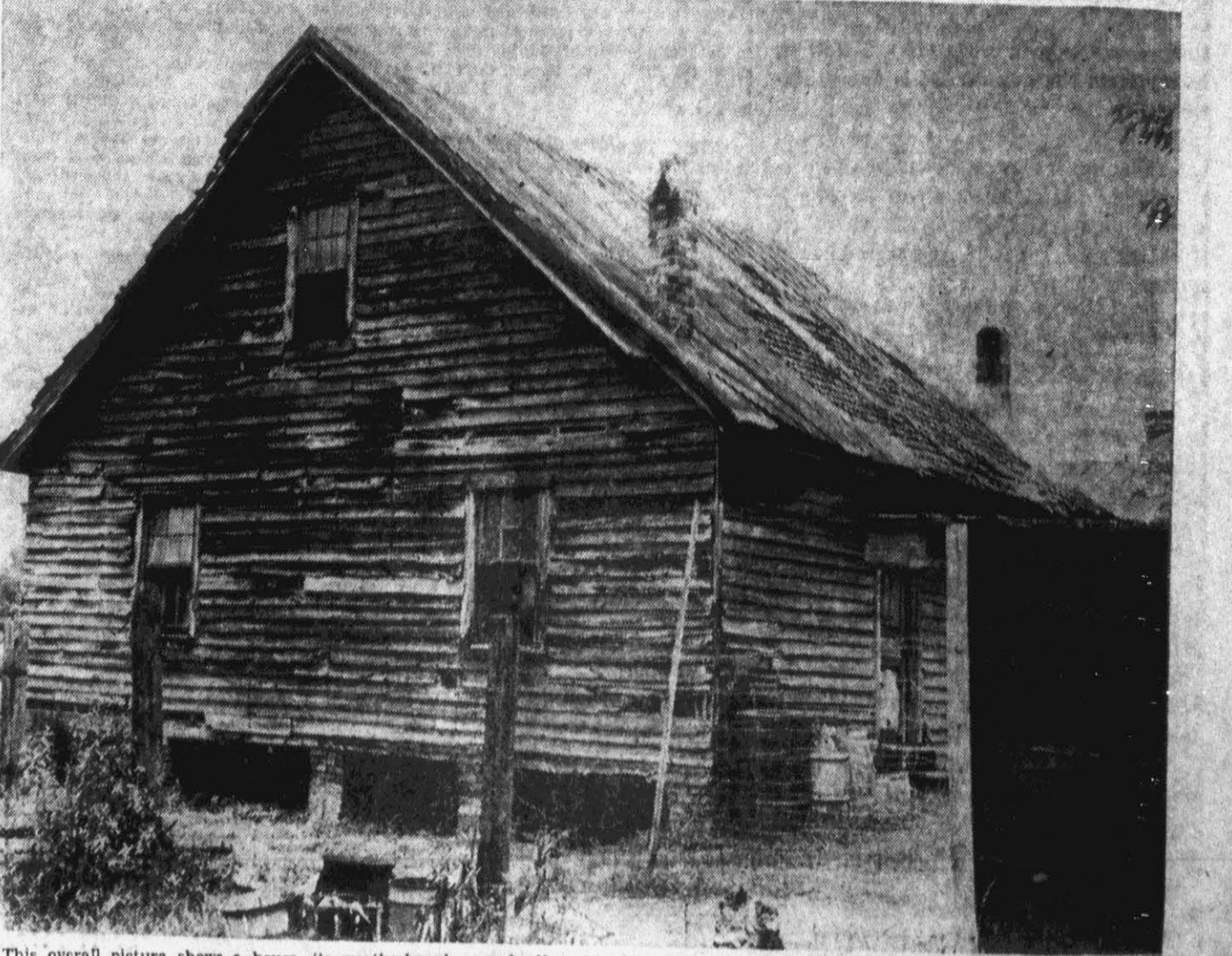
This overall picture shows a house, its weatherboard popped off and broken all over, exposing the walls on the inside of the house. Part of the roof is covered with tin while the other is not, allowing no shelter from the elements. A family of five live in this fire trap.
