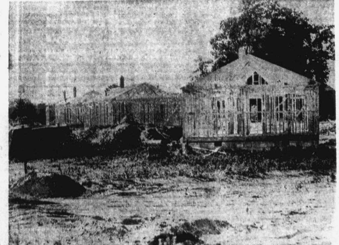
A total of 41 new houses are being constructed in the new housing project being built by Grifton Homes, Inc. The project will cost approximately $225,000 and will have 16 two-bedroom houses and 25 three-bedroom houses. The houses will be available for DuPont employees and other new residents who move to Grifton. The houses are expected to be ready for occupancy by August 15.
