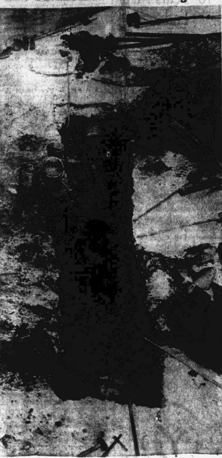
The above picture shows the hole which was cut in the floor of the Municipal Swimming Pool to uncover a broken sewer line lying some eight inches below the pool. The line broke recently causing raw sewage to enter the pool. The old sewer line was installed around 1905. (Reflector Staff Photo by Roy Hardee.)
