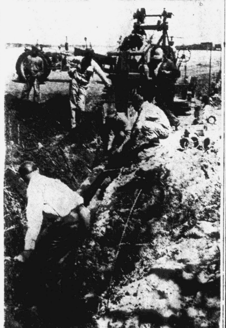
Many Pitt farmers have learned the value of having their wet and useless land turned into profitable, useable land, by tile drainage supervised by the soil conservation service. Here, workers prepare to put in place the pipe which will carry the water from the tiles into a canal. The tile-laying machine is shown in the background.
