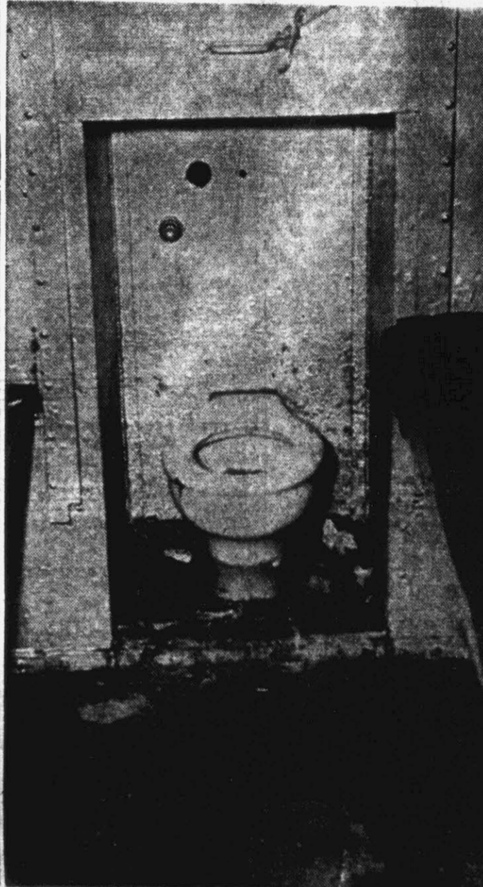
Part of the work toward renovating the county jail will go into new plumbing which marks the highest single item in the overall contract. In the picture above the floor around the toilet has completely rusted through two steel plates during the past several years. The toilet is used by the four occupants of the cell. (Photo by Roy Hardee).
