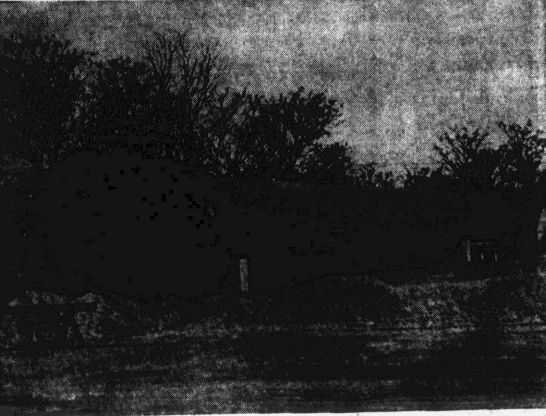
The gas tank shown above has been installed to help relieve the present low gas pressure in the southwestern area of the city. The 30,000 gallon steel cylinder was recently installed just off the Atlantic Coast-line railroad track between 12th and 13th streets. However, the recent railroad strike has held up shipment of parts that will complete the construction of the auxiliary pumping station. It is expected by the Utilities Commission that a 10-15 day waiting period will be necessitated before the station begins operation after arrival of the parts. (Staff Photo by Roy Hardee).
