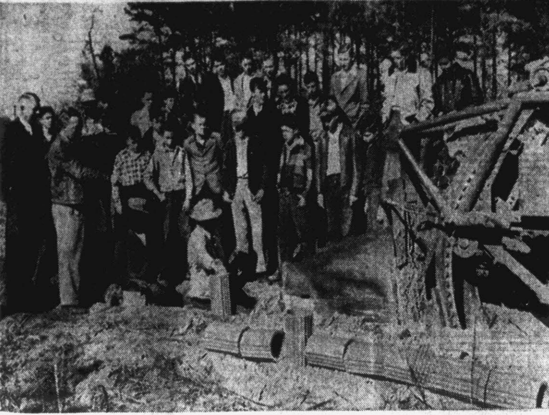
Members of the Winterville Agriculture class are shown as they watched a section of farm tile being put in place on the farm of Mrs. J. T. Gaylor of Winterville recently. The farm tile is being used to convert the wet, unusable land into fertile, profitable farm land showing the boys the tile operation and explaining it step by step is W. C. Eagles, of the Pitt Soil Conservation department (second from left, front). The class visited the project as a part of their study in farm conservation. (Reflector Staff Photo by Roy Hardee).
