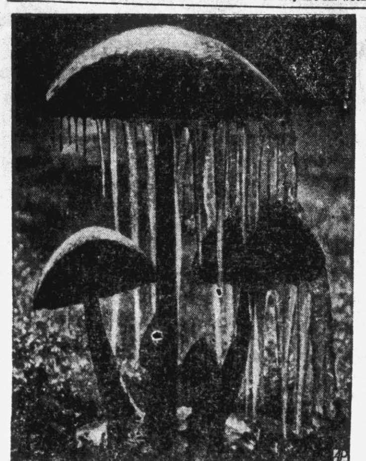
ICED MUSHROOMS — The underground sprinkling system on the lawn of W. D. Gridley's home in Tulsa, Okla., chose 24-degree-above-zero weather to break loose and coat these ornamental concrete outlets with thick layers of ice—and long icicles.
