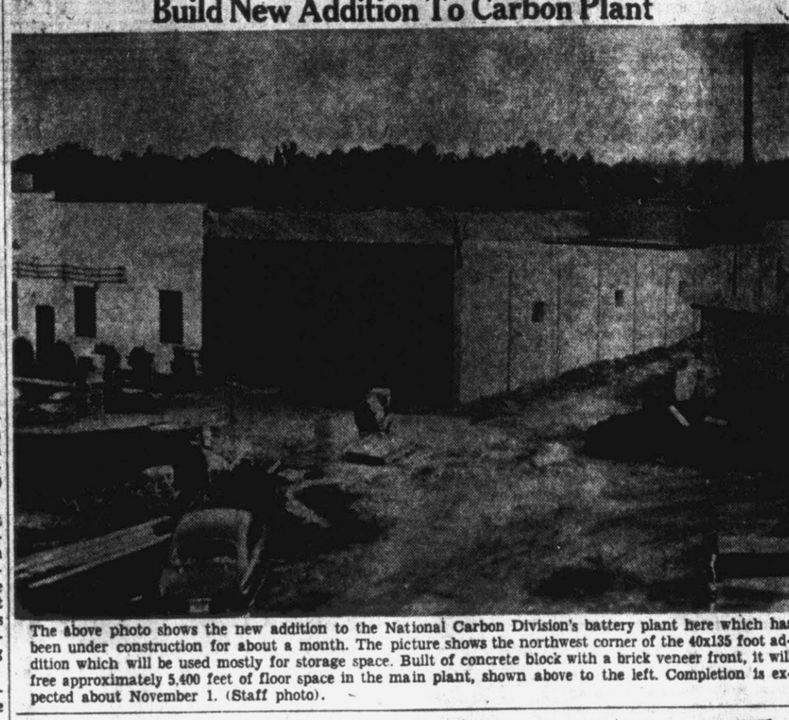
The above photo shows the new addition to the National Carbon Division's battery plant here which has been under construction for about a month.
