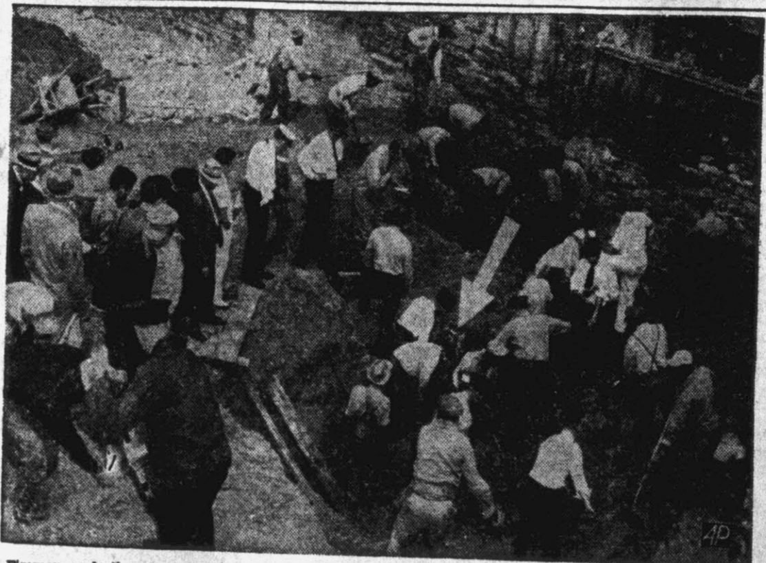
Firemen and other rescue workers dig in search of workmen buried under tons of earth and debris in the cave-in at an excavation project in downtown Atlanta, Ga., Friday. One worker was dug out and pronounced dead. Four others were believed buried alive. Six were dug out alive and taken to a hospital. The arrow points to the head of one worker who escaped burial completely by holding on to a board. (AP Photo).
