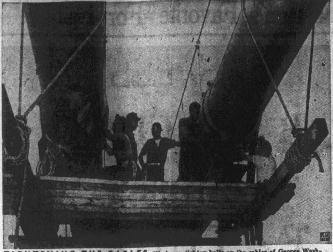
TIGHTENING THE CABLES —Workmen tighten bolts on the cables of George Washington Bridge between New York and New Jersey from a platform that will follow the span.
