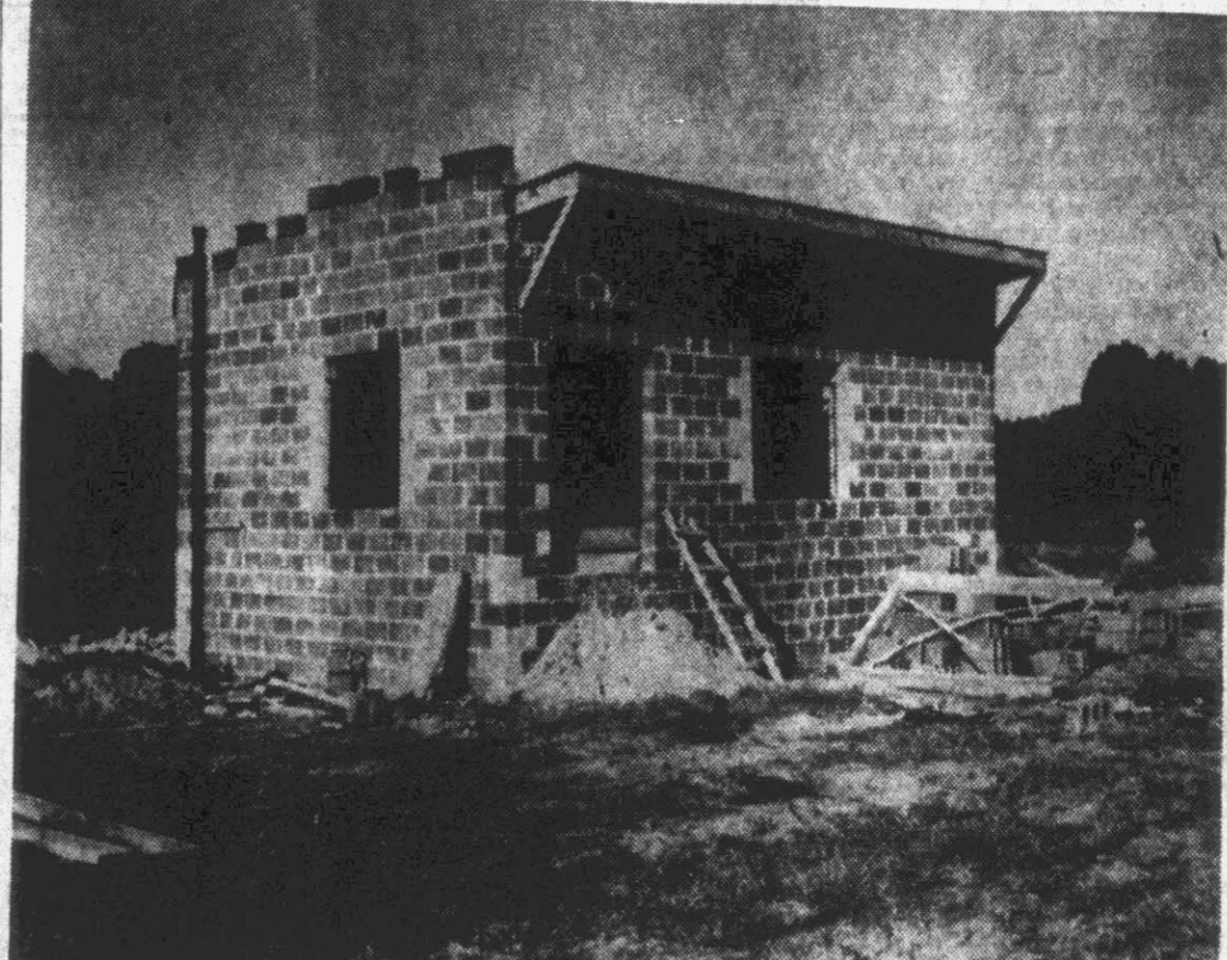
Rapid progress has been made on the construction of a new transmitter for Radio Station WGTC in the past several weeks. The building shown in the above photo will house the new equipment which will be needed to bring the local station's power up to 5,000 watts.
