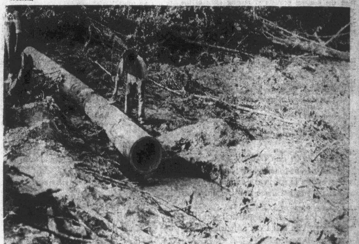
Bernie Wooten is shown installing a 15-inch concrete pipe, forty feet long through which will flow the surplus water that comes into a pond. The pipe when completed will rise above the surface of the pond about three inches. The pipe will take care of the needs of the pond under normal conditions, but in case of a flash flood, a sodded spillway has been built to carry off the water.
