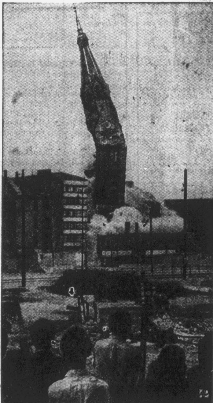
CHURCH STEEPLE BLOWN UP —The steeple of St. George's Protestant Church is blown up by an East Berlin demolition squad after Communists declared it a safety hazard.
