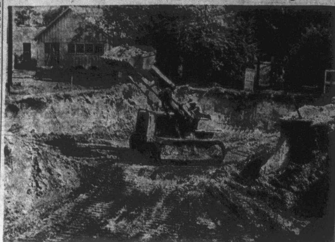
Work on the new Education building being built by the Jarvis Memorial Methodist church is rapidly coming along. Here a bulldozer begins to dig out the basement floor of the building. The building, when completed, will be one of the most modern buildings in every way. (Reflector staff photo by Roy Hardee).
