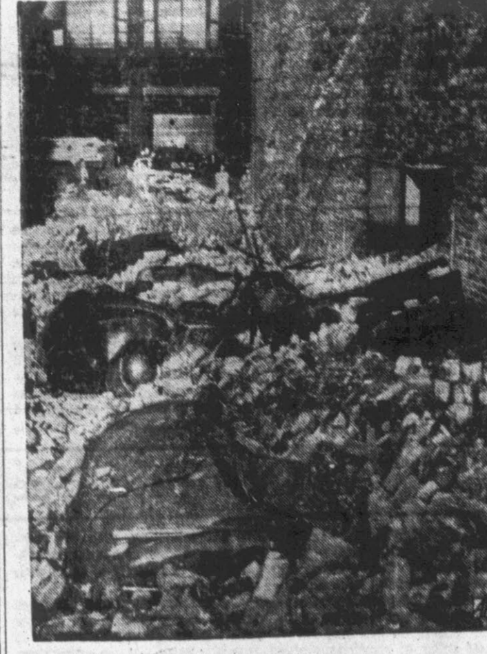
Tons of bricks from a three-story wall showered into this Chicago parking lot Saturday crushing seven cars and damaging four others. Army Sgt. Ike Thornton of Athens, Ga., had just driven his new 1950 car three miles from the salesroom to the lot when the wall fell. Fire department officials attributed the wall's collapse to a 23-degree drop in temperature in 35 minutes. Damage was estimated at $16,000. No one was injured. (AP Wirephoto).
