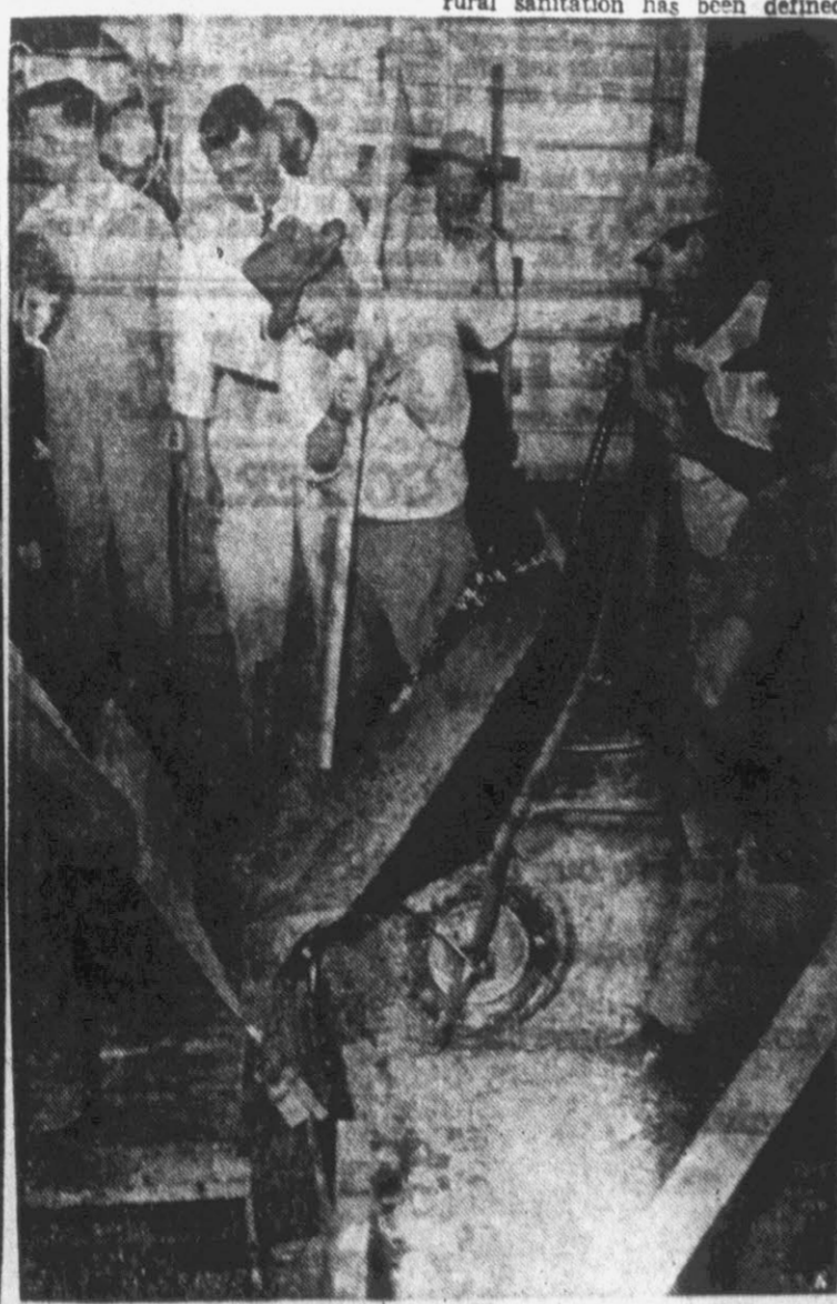
Part of the skeleton sanitation program in Pitt's rural areas is being undertaken in the above photo. Members of the vocational agriculture veterans group at Grimesland are shown above pouring cement into a septic tank wall form. The tank is one of the improvements one of the vets is making in his sewage disposal system. (All staff photos by Roy Hardee).
