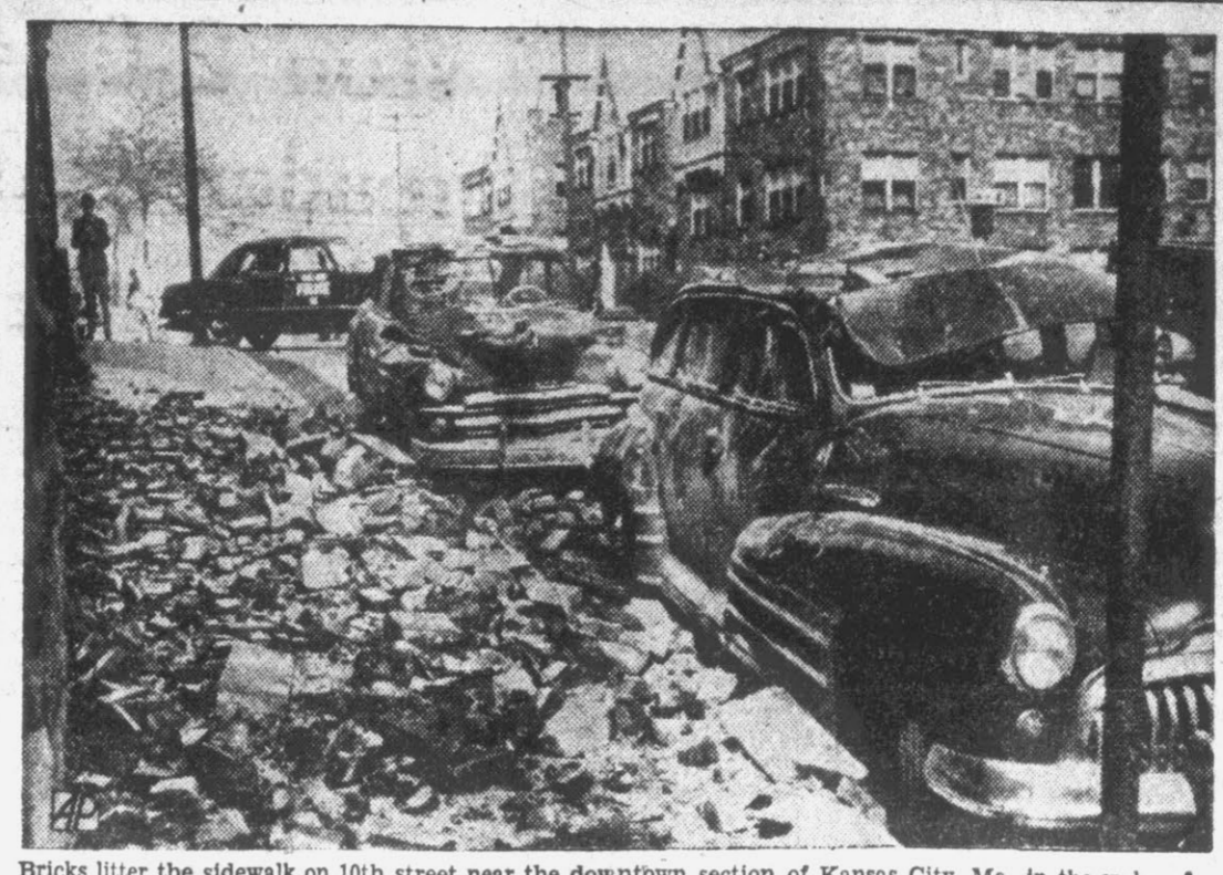
Bricks litter the sidewalk on 10th street near the downtown section of Kansas City, Mo., in the wake of a 70-mile-an-hour wind. This debris came from the top portion of a wall to a three-story apartment building. Two automobiles parked at the curb were damaged by falling bricks. Tornado winds cut a destructive path across parts of West Texas, Oklahoma and Kansas, killing at least one person and injuring about 50. (AP Wirephoto).
