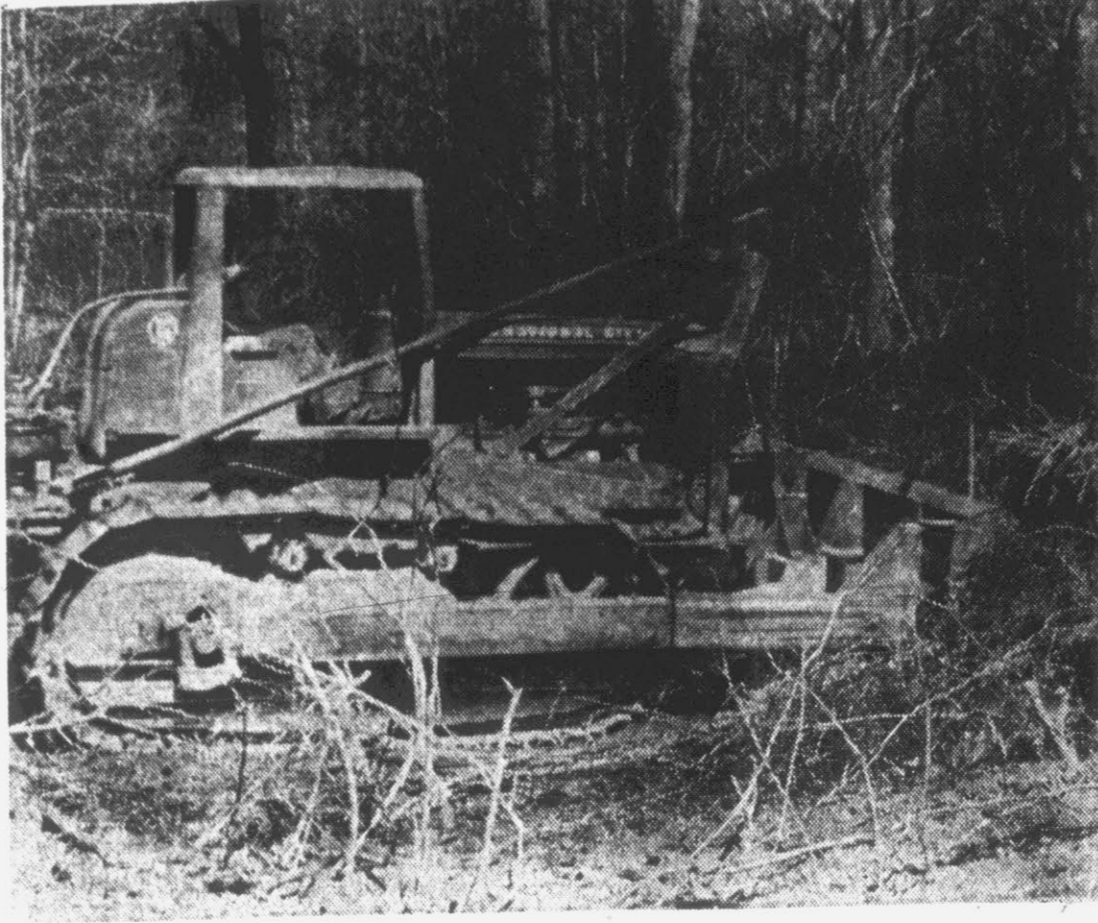
A bulldozer shown in the top photo is busy clearing land on the site of the new State Highway Patrol office building and garage which will be built at the intersection of the Tenth street highway. Bids for the construction of the buildings will be advertised in the near future, patrol officials have stated. (Reflector staff photo by Roy Hardee).
