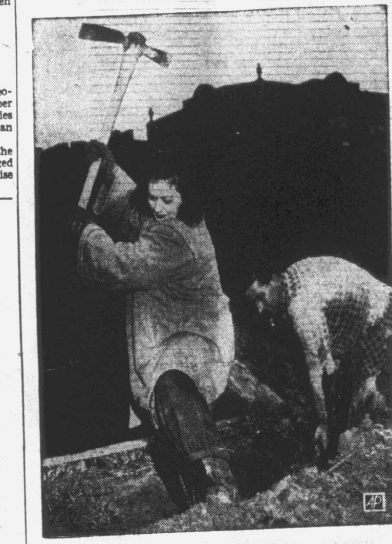
Mrs. Margaret Pallas, 22, divorcee and former office worker, swings a mattock in digging a ditch on a construction job in Chicago. She works an eight-hour day, digging, mixing cement and carrying pipe, and receives a daily wage of $10. Behind Margaret is her boss, Donald Buss, 31, a contractor, who says they plan to get married. While she toils, relatives care for her two-year-old daughter. (AP Wirephoto).
