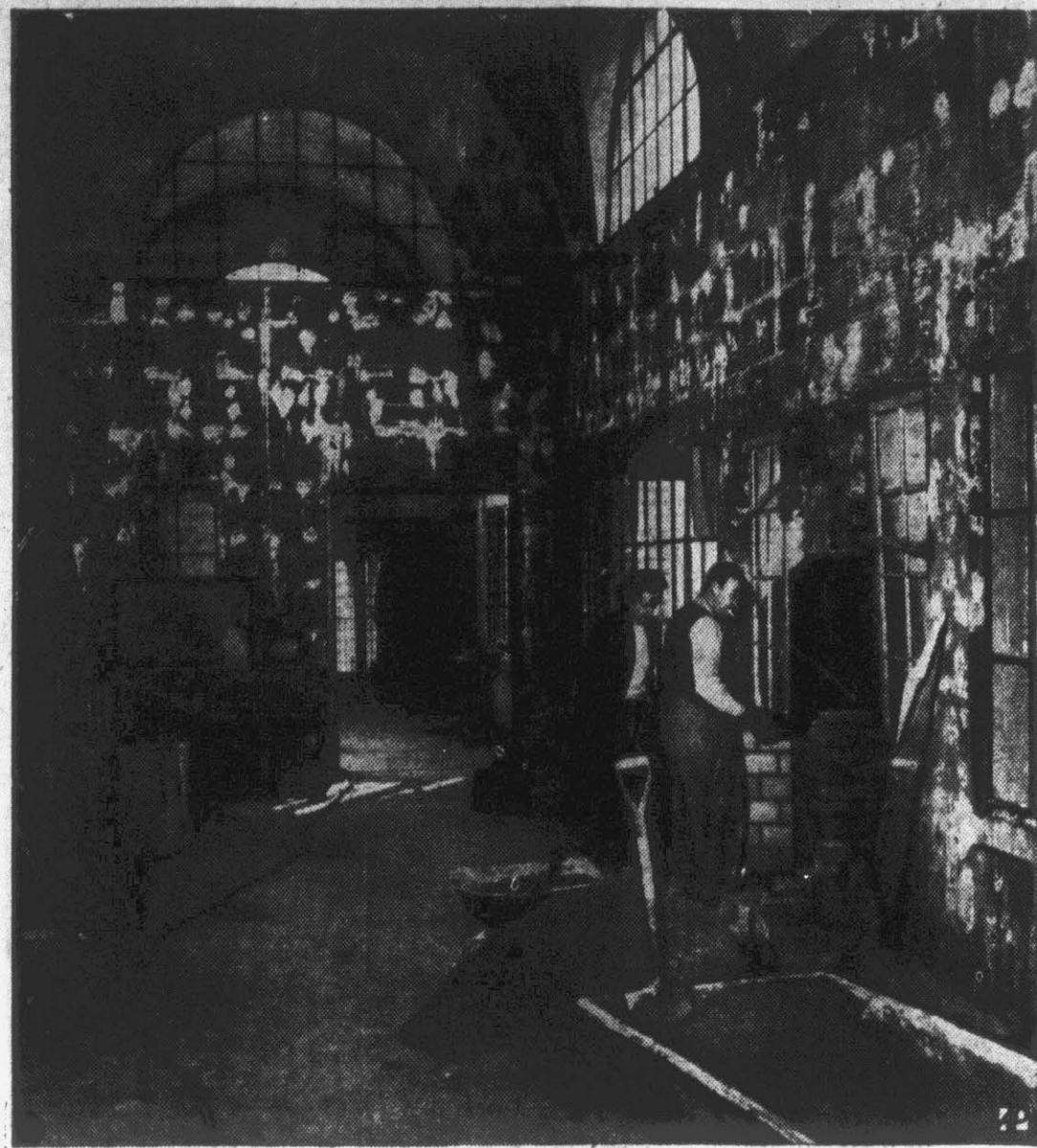
OLD STATION TO BECOME HOME—Miss C. Louise Pollet supervises fireplace construction in abandoned railway station she is converting into a home at New Rochelle, N. Y.
