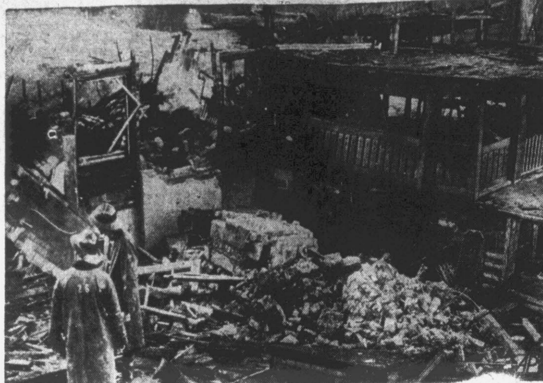
Five persons perished in this wreckage of an antique shop destroyed by a gas explosion at Birmingham, Mich. Two others were reported missing in the disaster. Firemen survey the ruins. Among the victims was a fire prevention expert from the Birmingham fire department who had been called to the shop to investigate a gas leak. (AP Wirephoto).
