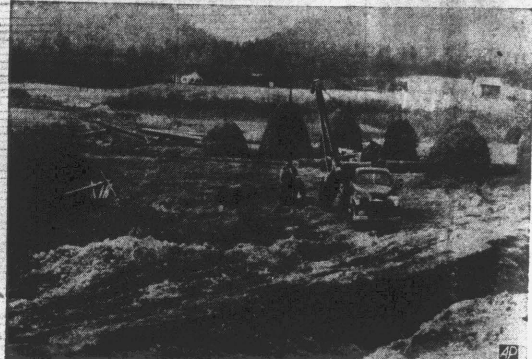
Employment of non-union workmen such as this crew is blamed in some quarters for the wildcat strike that briefly halted construction of two gigantic atomic plants at Oak Ridge, Tenn. These nonunion men employed by the Olan Construction Company in laying a $10,000,000 pipeline from middle Tennessee to supply the atomic installations with natural gas. The strike of A.F.I. construction workers set off a chain reaction which idled more than 2,000 Oak Ridge employes. (AP Photo).
