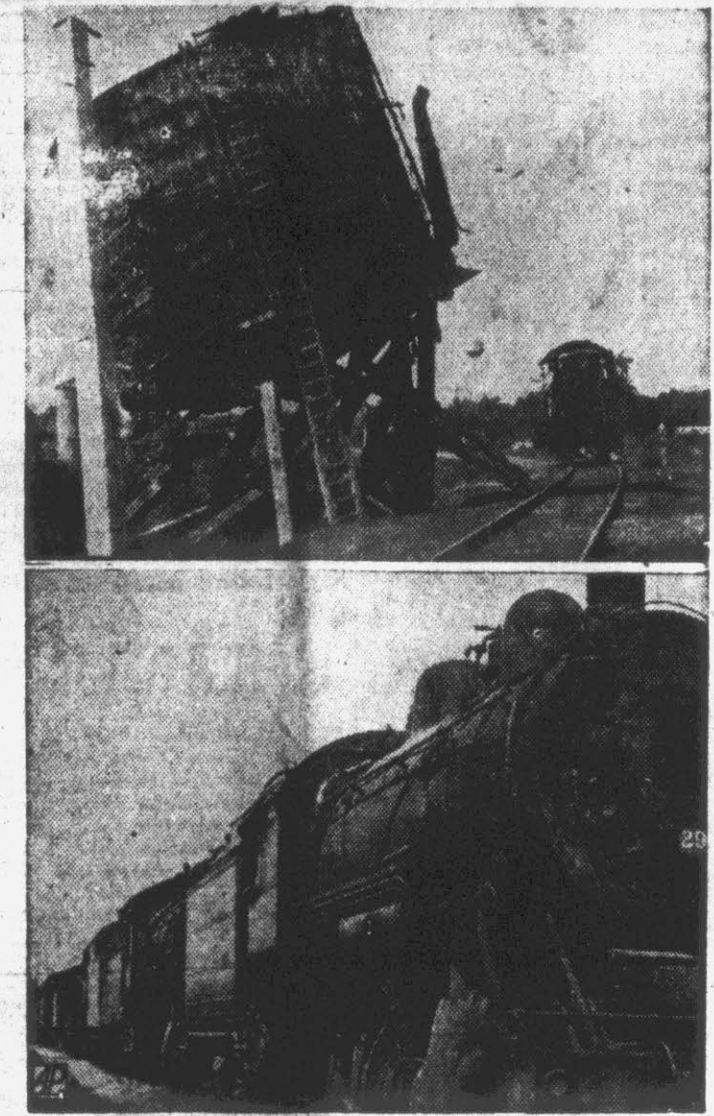
A 50-year-old water tank (top) is pulled down at Columbus, Miss., just after the last steam locomotive on the Gulf, Mobile & Ohio railroad had finished its final run. This winds up the railroad's $60,000,000 modernization program in which all of the old steam engines have been replaced with modern Diesels. Diesels don't need water, and so the tanks are being razed. At the bottom are some of the G. M. & O.'s 300 steam locomotives in a "graveyard" at Jackson, Tenn. They are being converted into junk. The G. M. & O. claim to be the first major trunk line railway in the nation to achieve complete dieselization. (AP Photos.)
