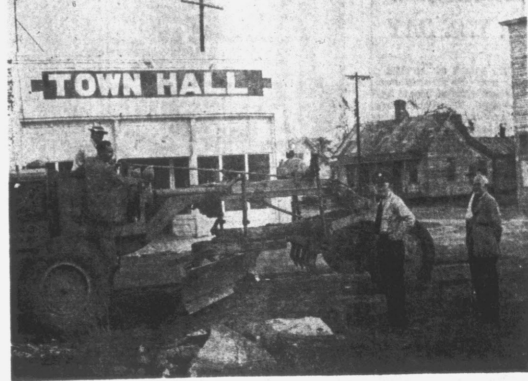
This grader is putting the finishing touches on the shoulder of the newly paved street which runs in front of the Winterville town hall. Woodrow Worthington, one of the leaders in the paving project, has climbed up on the machine with Operator F. L. Satterthwaite to see how the job is done, while Police Chief Buck, F. A. Worthington and F. A. McLawhorn look on. (Daily Reflector Photos).
