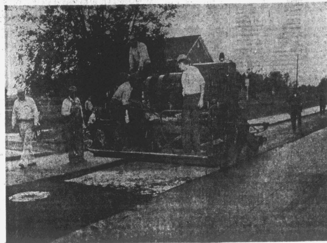
The paving machine is putting the middle lane in one of Winterville's new streets. In October the town had only two blocks of paved streets in addition to the state highways. Today there are approximately 35 blocks of paved streets in the town.
