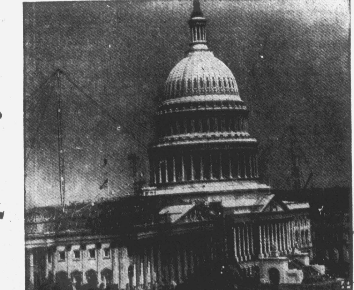
CAPITOL UNDERGOES REPAIRS—In midst of derricks and scaffolding, workmen repair Capitol roof at Washington. House and Senate chambers will be completed in December.
