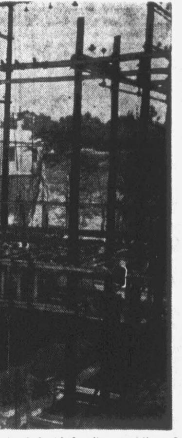
The power plant sub-station controls all the power produced at the local plant before it goes out through the lines into the city. (Staff photo by Roy Hardee).
