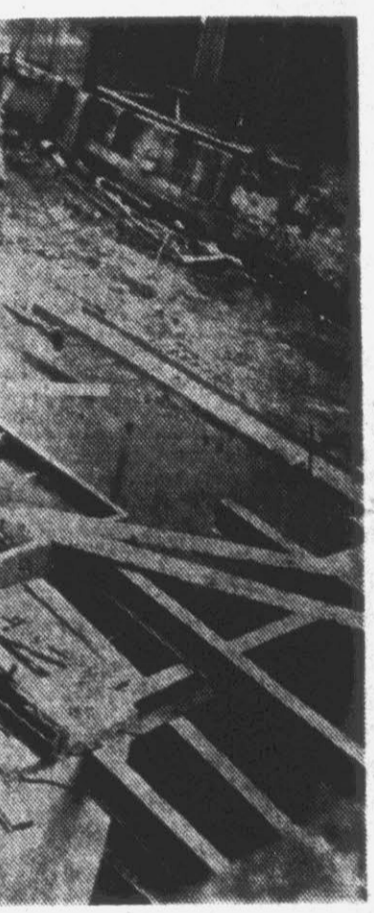
Workers are constructing the bottom section of the building which is being built to house the new 5,000 kw generator.
