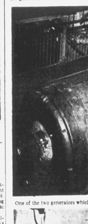
One of the two generators which are supplying electric power for the Greenville area is pictured above.
