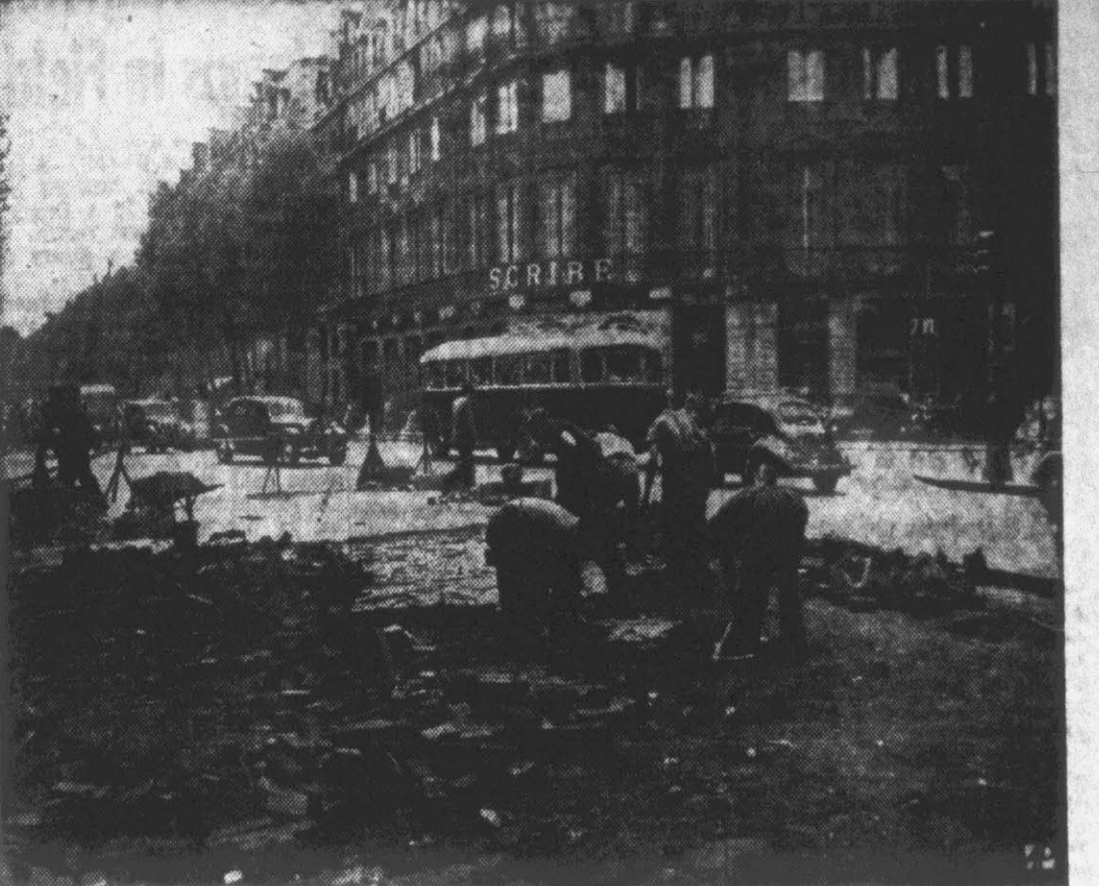
PARIS TEARS UP WOOD PAVEMENT —Workmen take up wood blocks on the Boulevard des Capucines, Paris, to replace them with bricks and asphalt, safer for autos when wet.
