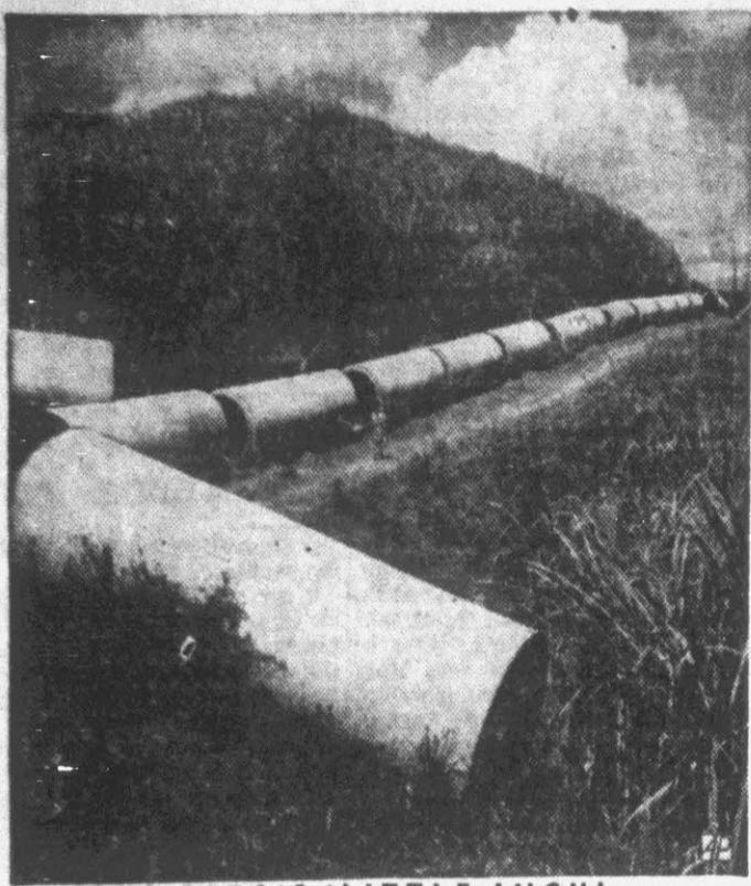
PUERTO RICO'S 'LITTLE INCH' —Sections of Puerto Rico's "Little Inch," $25,000,000 San Juan water system, line the route from filtration plant to the reservoir.
