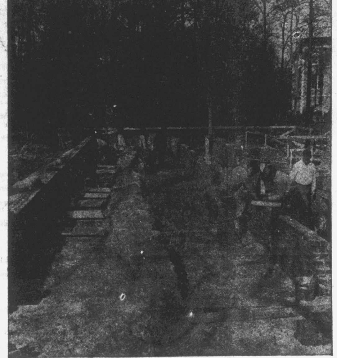
Work is progressing on Slay Hall, new dormitory for men students now being erected on the campus of East Carolina Teachers College. Ground was broken for the new building November 15 by Ralph M. Garrett of Greenville, chairman of the building committee of the college Board of Trustees. Shown above are workmen busy on the construction of the residence hall, which will provide living quarters for 216 of the approximately 700 men students at the college. The new building was recently named by the Board of Trustees in honor of the late Dr. Ronald J. Slay, for 22 years head of the department of science at the college and its first dean of instruction. Slay Hall is located in a grove of trees on the campus and will be situated near Ninth street.
