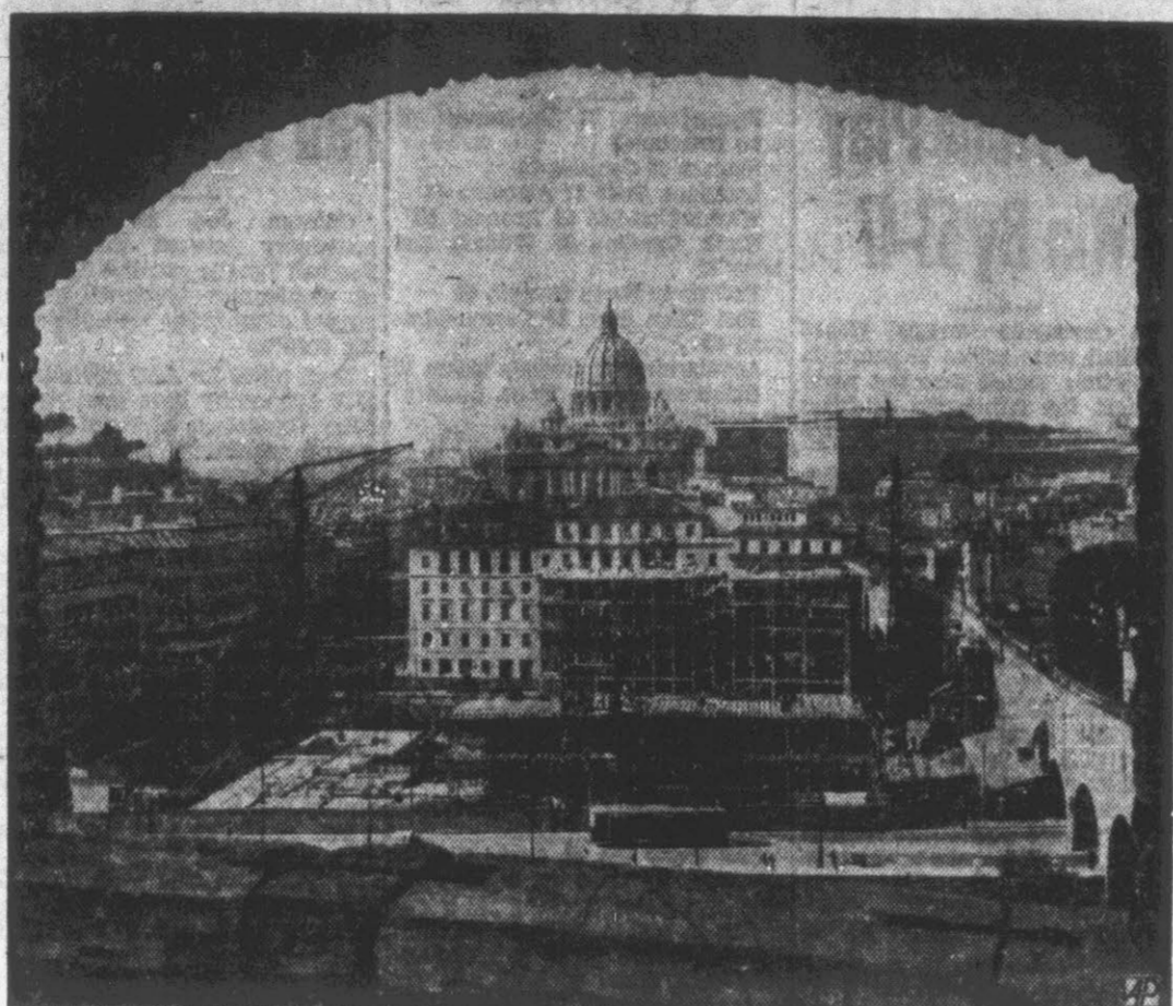
HOTEL FOR PILGRIMS —The building (foreground) being constructed near St. Peter's (background) in Rome will house pilgrims who will visit the city during Holy Year of 1950. Offices of Catholic Action groups will be in the building.
