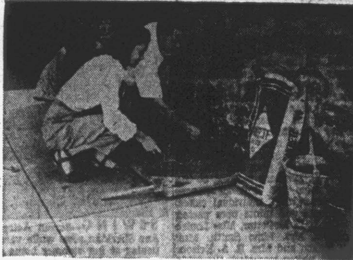
See how easy it is to patch a wall with SAKRETE Mortar Mix. Walls should be repaired before small cracks become big breaks.
