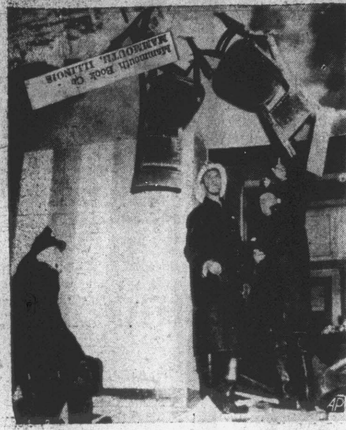
These chairs were imbedded in the second floor ceiling in a three-story downtown building in Buffalo, N. Y., by an explosion which wrecked the building, January 12. Two persons were cut by flying glass in the building, which was owned and occupied by Unterecker's, Inc., a candy firm. (AP Wire photo).
