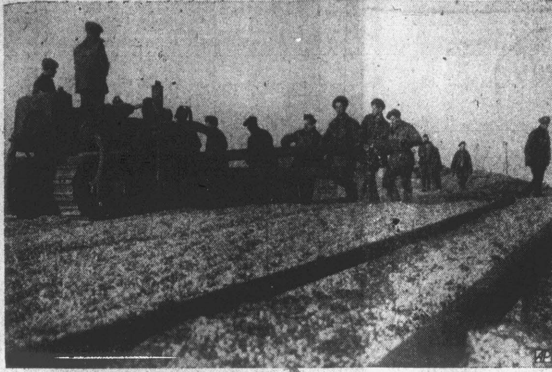
PLUTO'S SECRETS REVEALED—Bulldozers carry away heavy pipelines which conveyed petrol to Pluto, submarine line from Dungeness, England, to France, which is being dismantled. Pluto supplied Allied forces during the invasion of Normandy. The secret of the line was so well kept that only now are people living in Dungeness learning of its presence.
