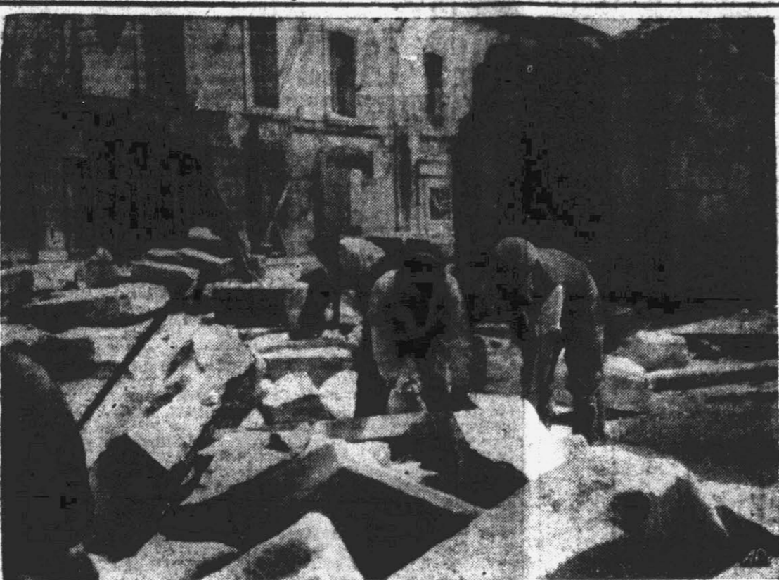
'REBUILDING' ST. MALO —French civilians in St. Malo bend to the task of reconstructing their historic old city, badly damaged during the war.
