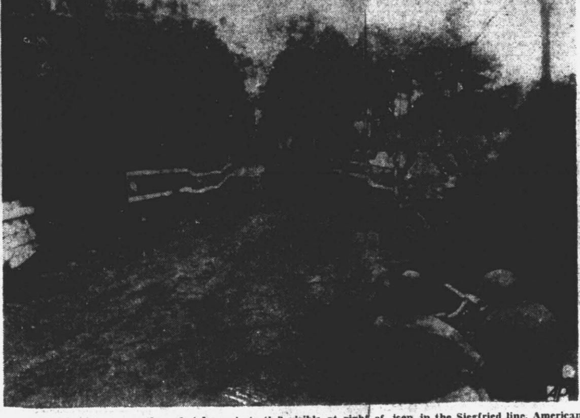
After clearing a way through "dragon's teeth," visible at right of jeep, in the Siegfried line, American engineers man a machine gun to guard a small bridge they have constructed in Germany. (AP Wirephoto from U. S. Army Signal Corps).
