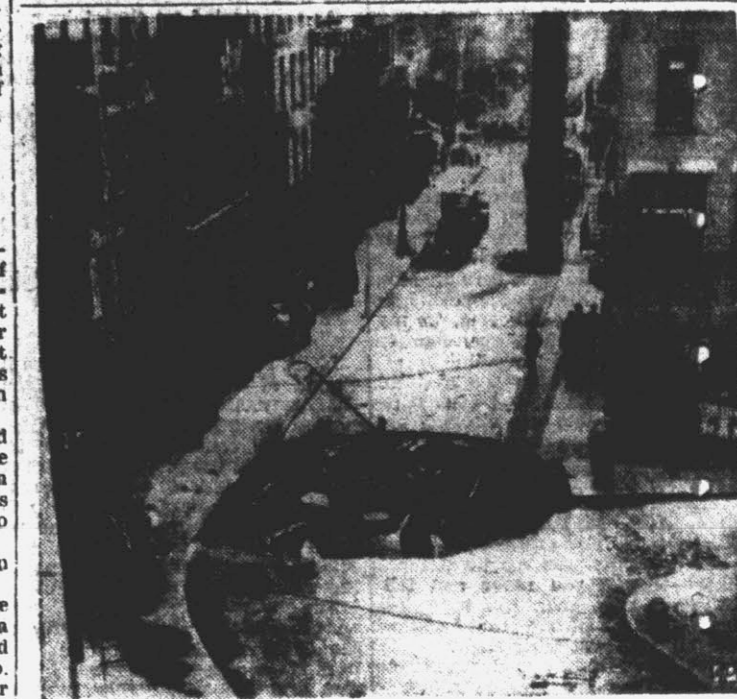
NO, NOT A BOMB —A water main break and gas explosion, not enemy action, made this hole in the paving at Mott and Pell streets, in the heart of New York's Chinatown.
