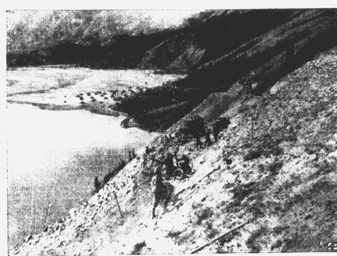
HILLSIDE HIGHWAY—Using compressed air and pneumatic tools, U. S. Army Engineers cut a roadway into the steep side of a hill. Note their bivouac in background.
