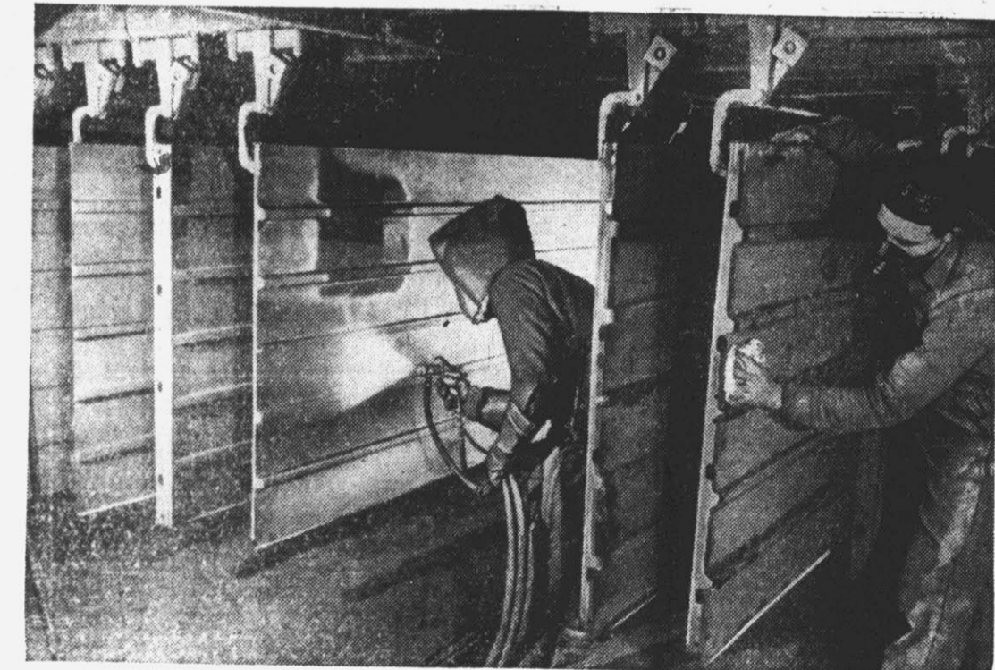
The story of the prefabricated house begins at the factory where its parts are turned out on a mass production basis. These workmen are applying paint to steel panels preparatory to shipment.
