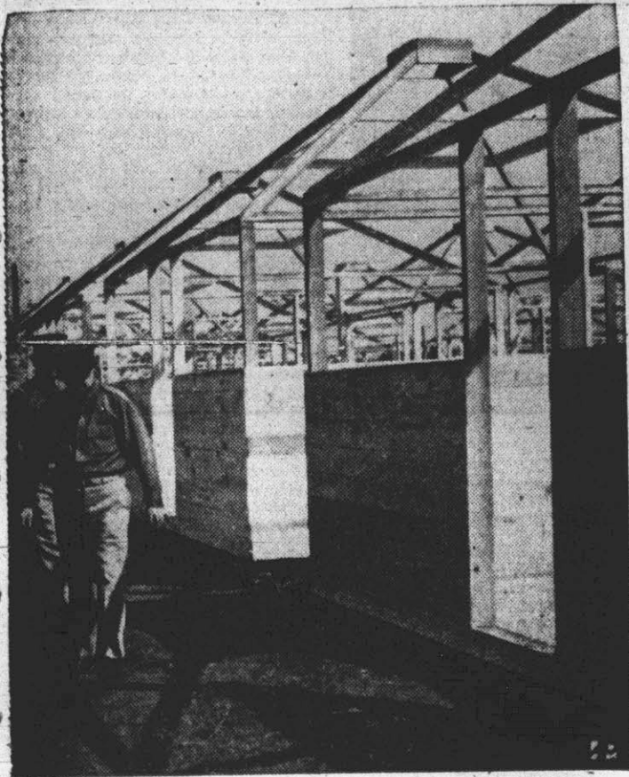
ARMY 'FRAMEUP' —Typical of frames over which tents will be stretched are these army buildings at Yaphank, L. I.
