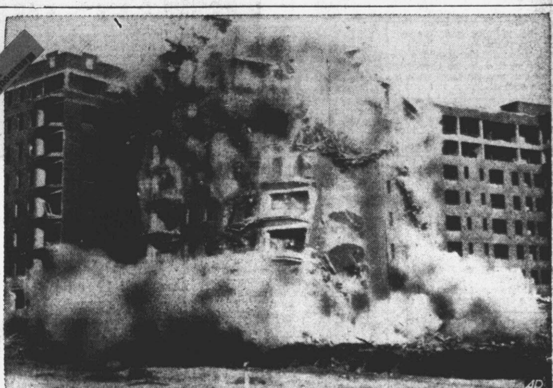
The capital city of Washington was subjected to a planned "bombing" when one wing of the $2,000,000 Boulevard apartments was dynamited to make way for the $4,000,000 first unit of the proposed $26,000,000 War Department building. This picture was made just as the dynamite exploded and the walls of the nine-story building began crumbling.
