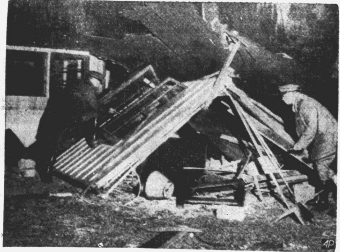
Two women were hurled 40 feet to their death and six other persons were injured by the explosion of two small tanks used for heating water which partially demolished the home of John Kimmer near Savannah, Ga. Those who perished were Kimmer's wife and Mrs. Alberta Richardson. County policemen are shown searching the wreckage shortly after the explosion.
