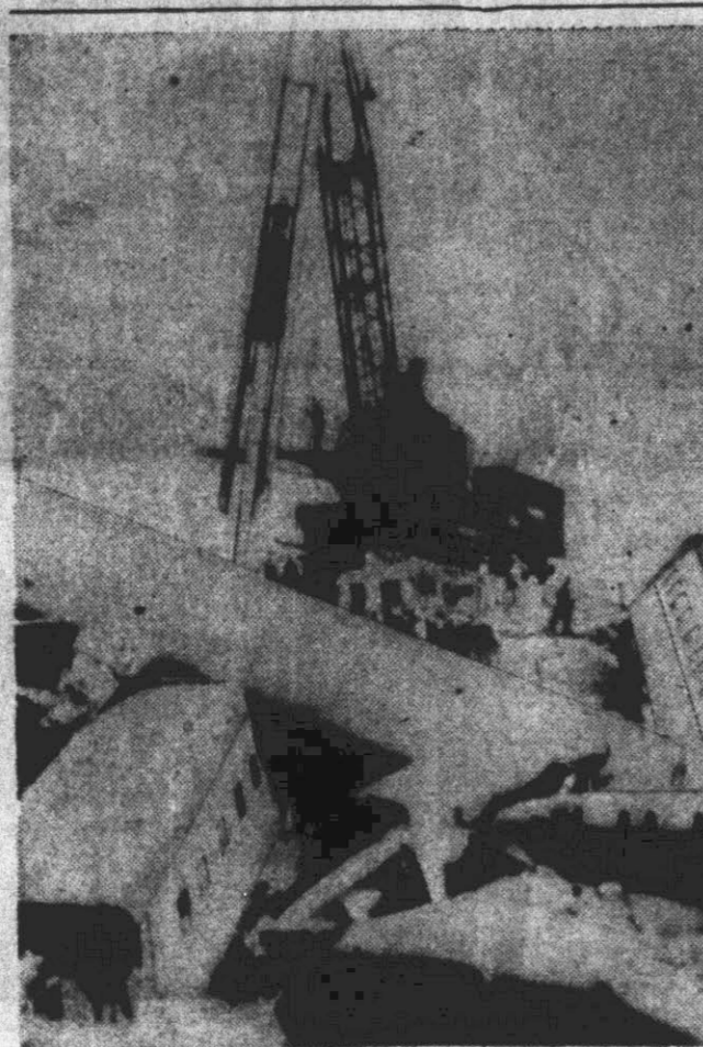
While investigators sought the mysterious person believed to be earless, who was responsible for the "key of San Francisco" train wreck in central Nevada, it fell to railroad men to go ahead with the tremendous salvage task. This picture shows a pile driver in the midst of the wreckage at work rebuilding the Humboldt river bridge.
