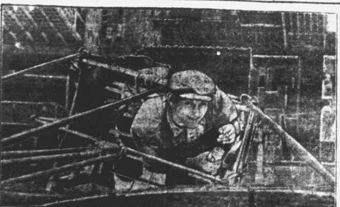
ONE HUNDRED AND ONE STORIES UP: Sidney Evert, glazier, "lets up and lights up" while repairing broken glass outside the hundred and first floor of the Empire State Building, New York City. He's more than 1000 feet above the street.
