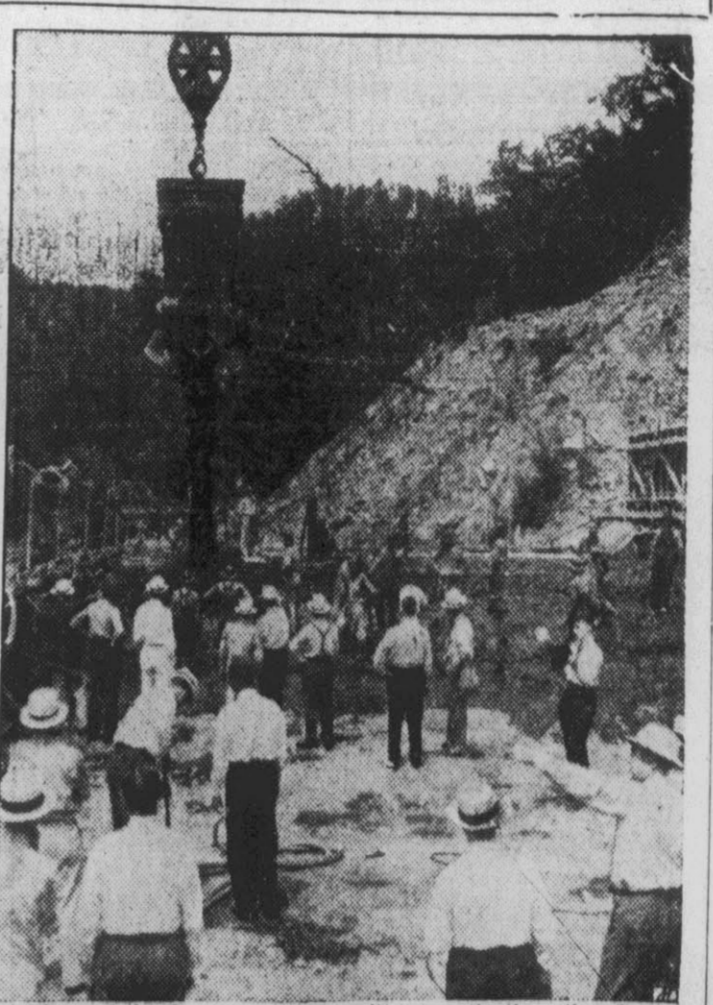
Members of the Congressional committee investigating the Tennessee Valley Authority showed considerable interest in the operation of this huge crane as they stopped at Hiwassee dam in North Carolina to inspect one of the TVA's newest projects. Hiwassee was the first stop on an 800-mile tour of various TVA dams.
