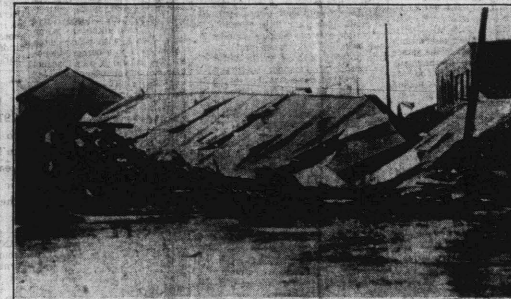
The above wooden structure at Goulds, Fla., was wrecked by strong winds accompanying a tropical disturbance that swept the Florida Keys. (AP Photo.)
