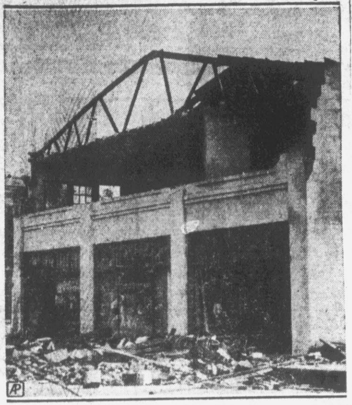
The West Indian hurricane which swept Florida caused untold damage in the business district of the little town of Stuart. This photograph shows the wreckage of an automobile company and a curio shop, which were in the path of the heavy wind.
