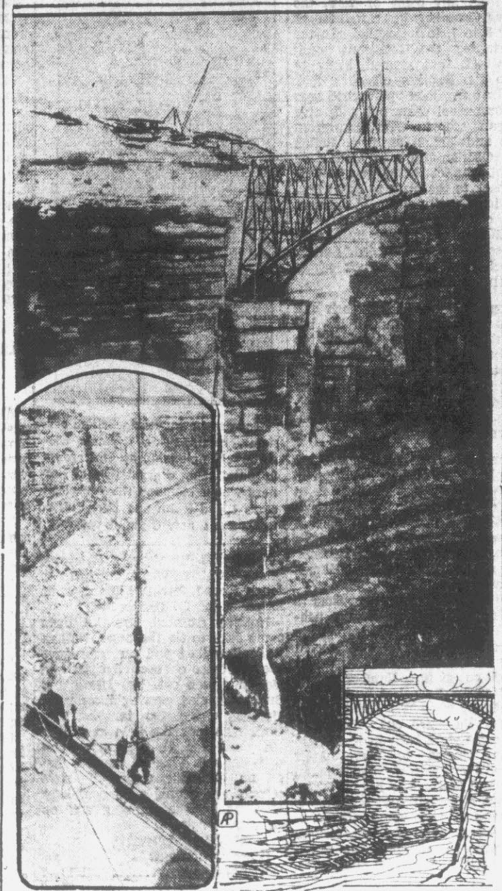
Opening a vast and little known region to tourists, a great bridge over the Grand Canyon and the Colorado River, shown above under construction, will be completed by Sept. 1. The inset, showing bridge workers at their task almost 500 feet above the water, suggests the great height of the span.
